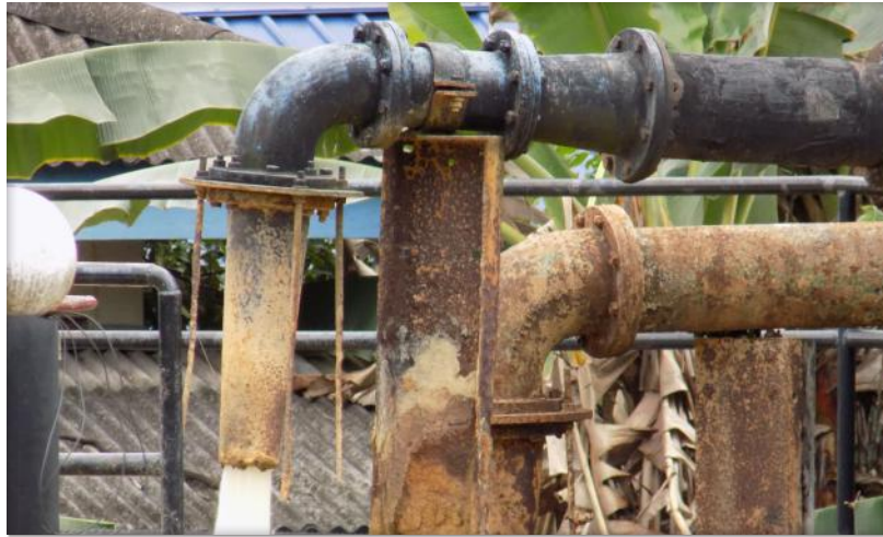
Figure 15. Pipes at a water treatment plant in Raub built in 1929. Photo Credit: Kara Runsten, 2017
